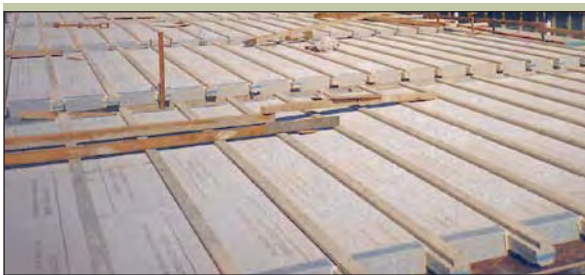
FIGURE 17: Ultrafloor composite floor system
